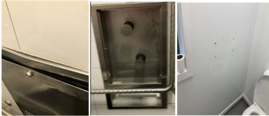
Figure 17 Photos of Broadway Toilets and Centennial Rest Room damage.
