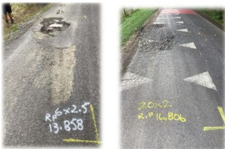
Figure 1: Pavement repairs required on Brewer Road outside Makahu School
