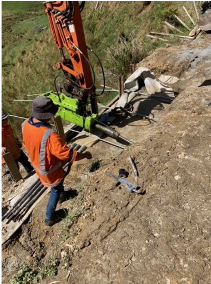
Figure 2: RP0.8 - Drilling the holes for the horizontal ground anchors to be installed.
