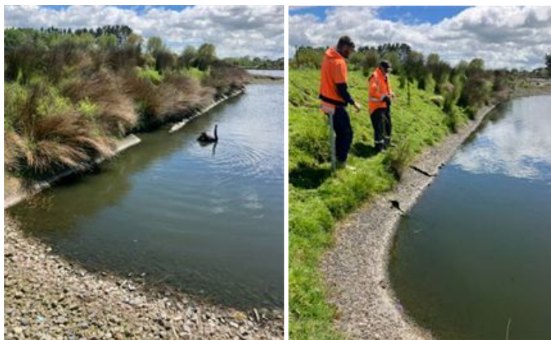
Figure 6: Wastewater Treatment Plant Pond wall damage
