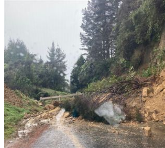
Above: A slip on Matau Road during a severe weather event in 2022.
