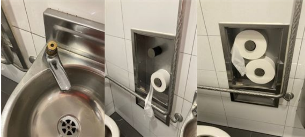
Figure 6: Photos of Broadway toilets missing toilet paper dispenser doors and accessibility tape
