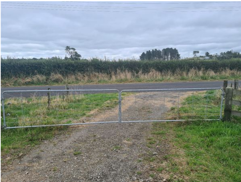
Figure 4: The other current outer gate onto the wastewater oxidation pond property, one side lacks electrified wire.
