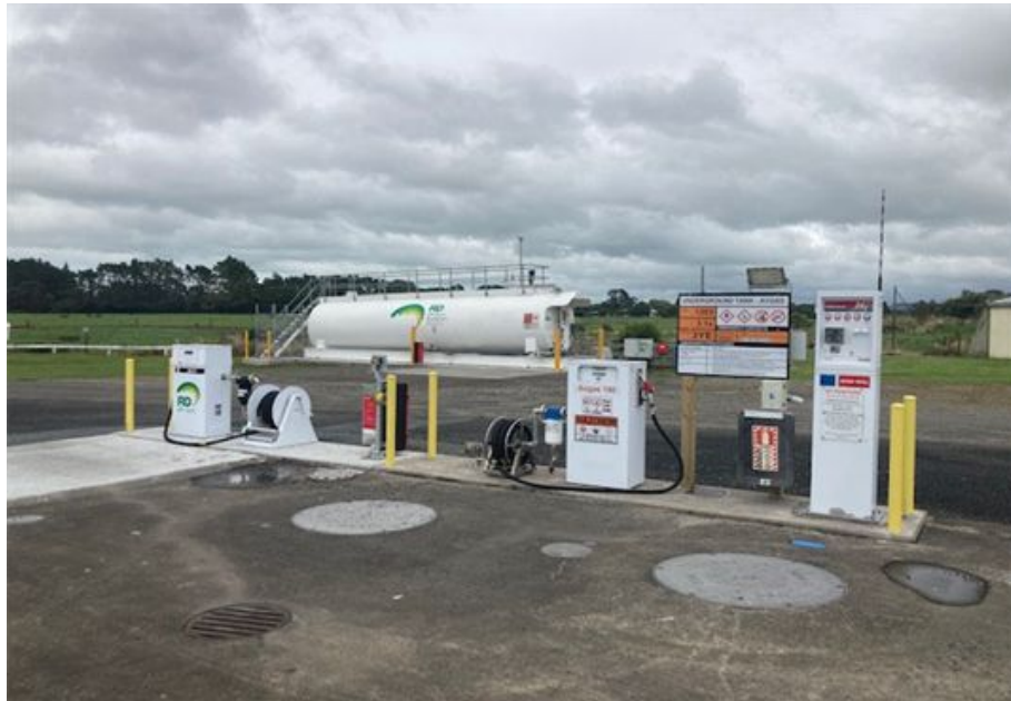
Figure 5: Completion Photo of RD Petroleum Jet A1 Fuel Tank and Dispenser
