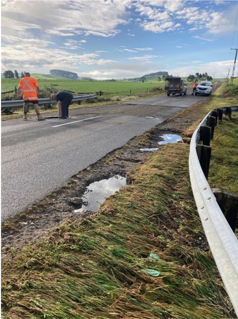
Figure 3: Seal damage on Oru Road
