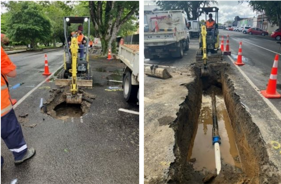
Figure 9: Water line failure on Fenton Street – AC pipe split
