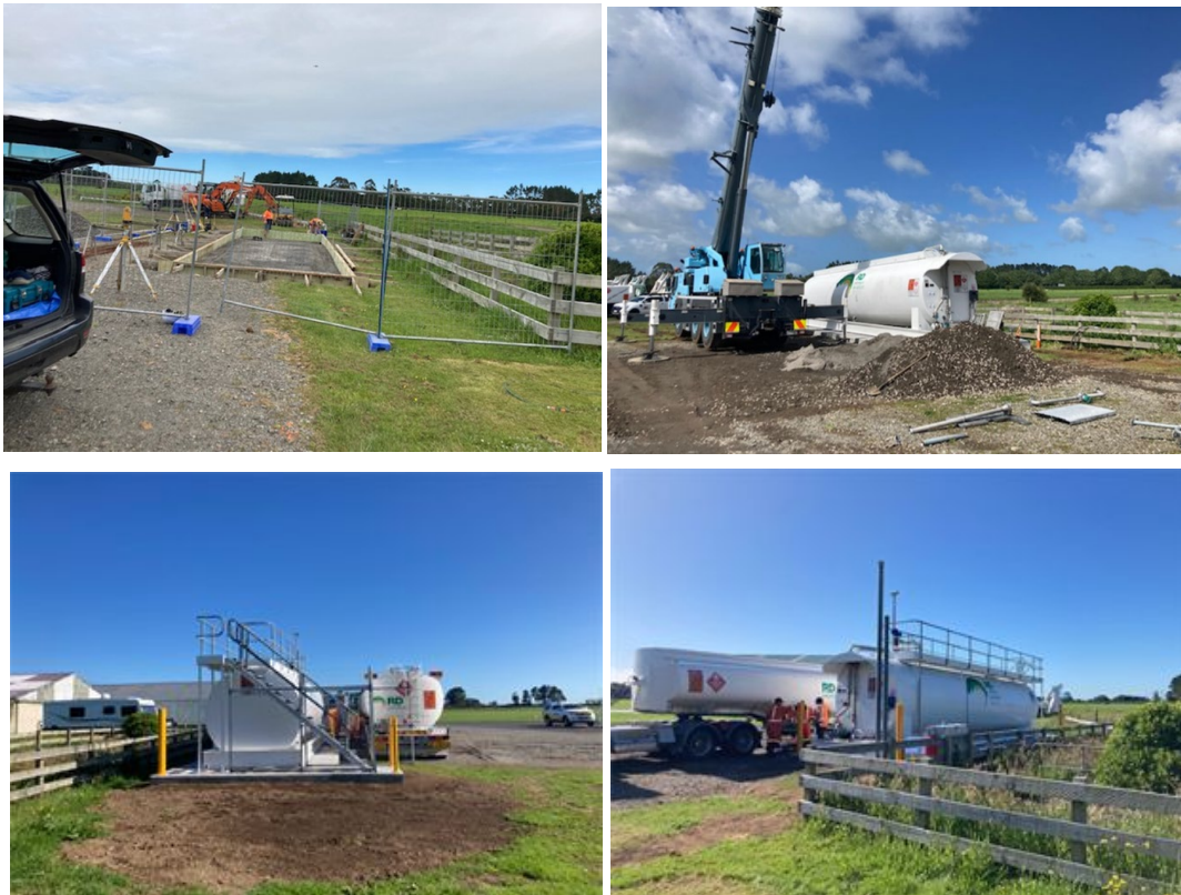
Figure 13: Progress photos of the installation of the RD Jet A1 Fuel Tank and Dispenser
