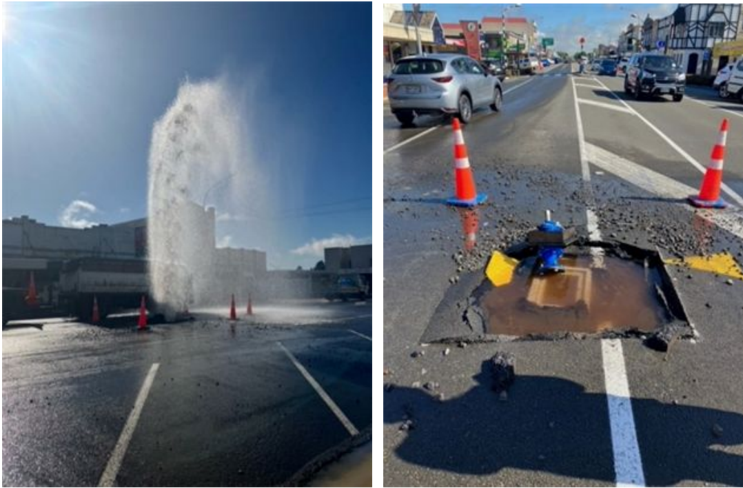
Figure 8: Mains break on Broadway – Hydrant failure after impact
