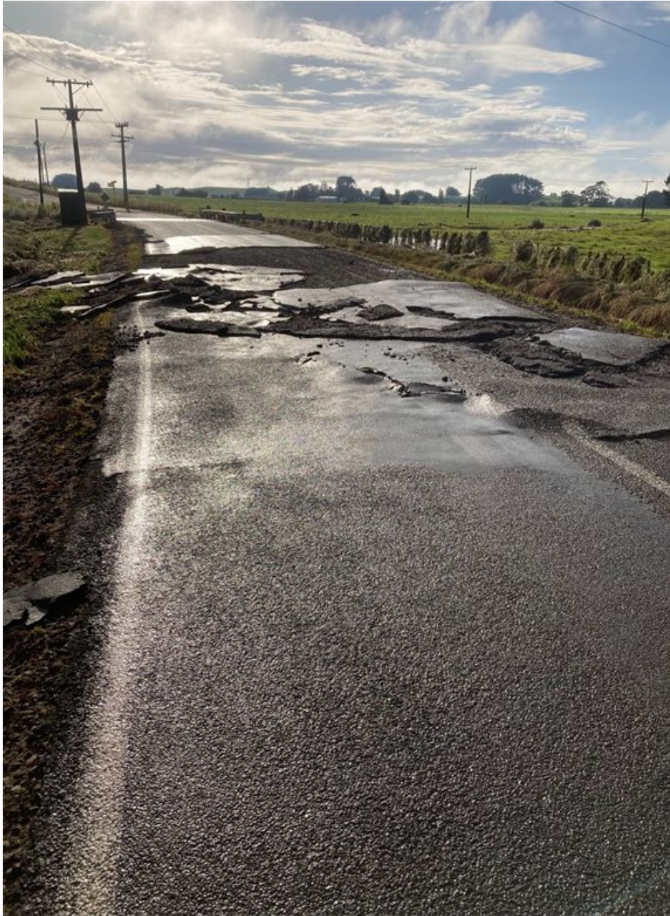
Figure 2: Damage caused to Cheal Road by the floodwaters
