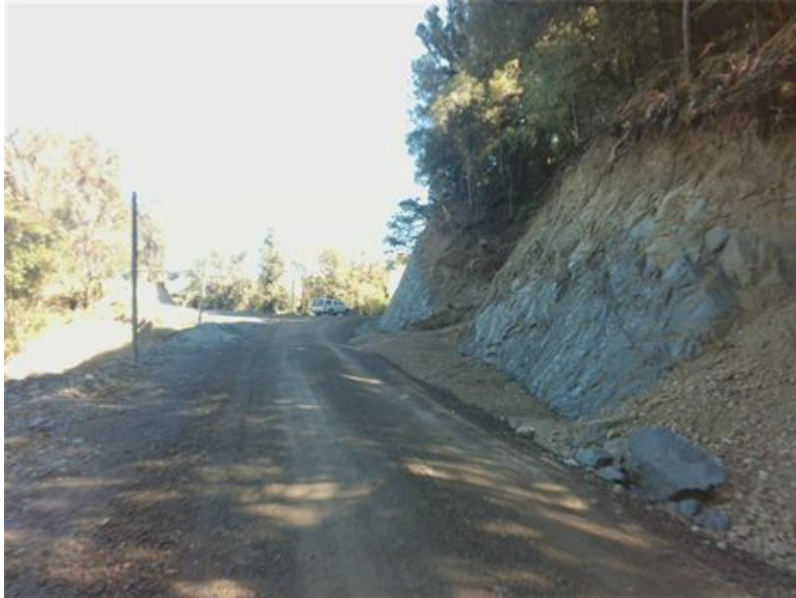
Figure 1: Bank retreat on Putikituna Road
