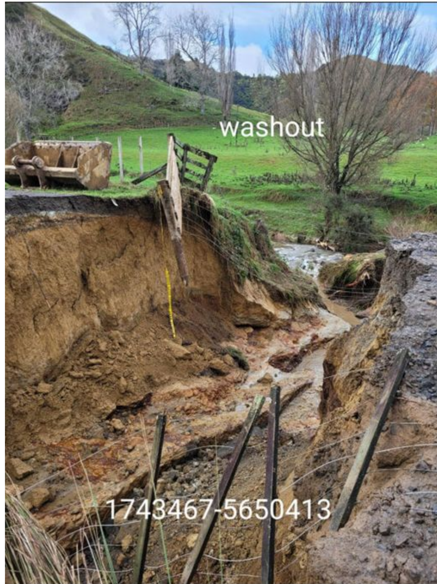
Figure 10: Upper Mangaehu Road. New Culvert and the road re-constructed. Cost of the works = $125,500
