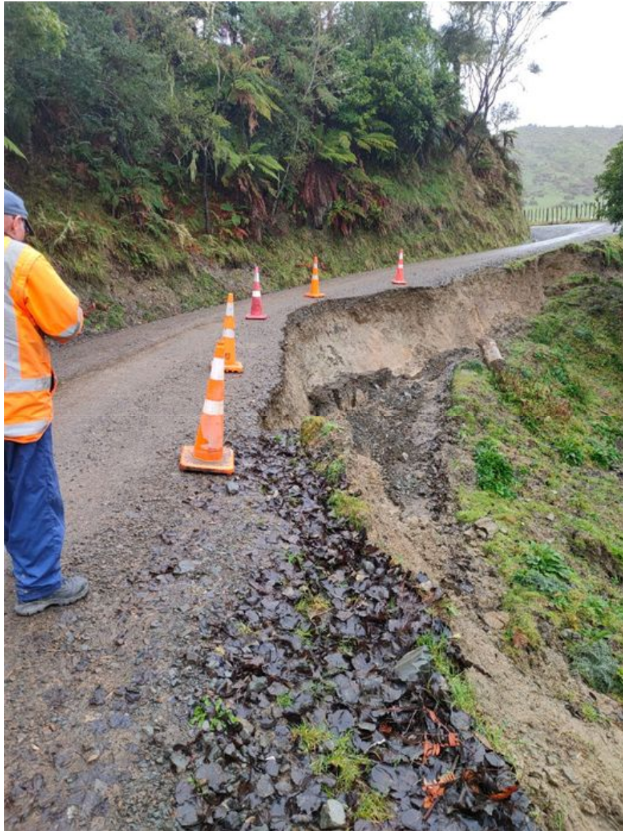
Figure 11: Lower Kohuratahi Road, most likely a retreat into the bank, including the removal of the curve in the distance. Estimated costs $50,000 - $80,000.
