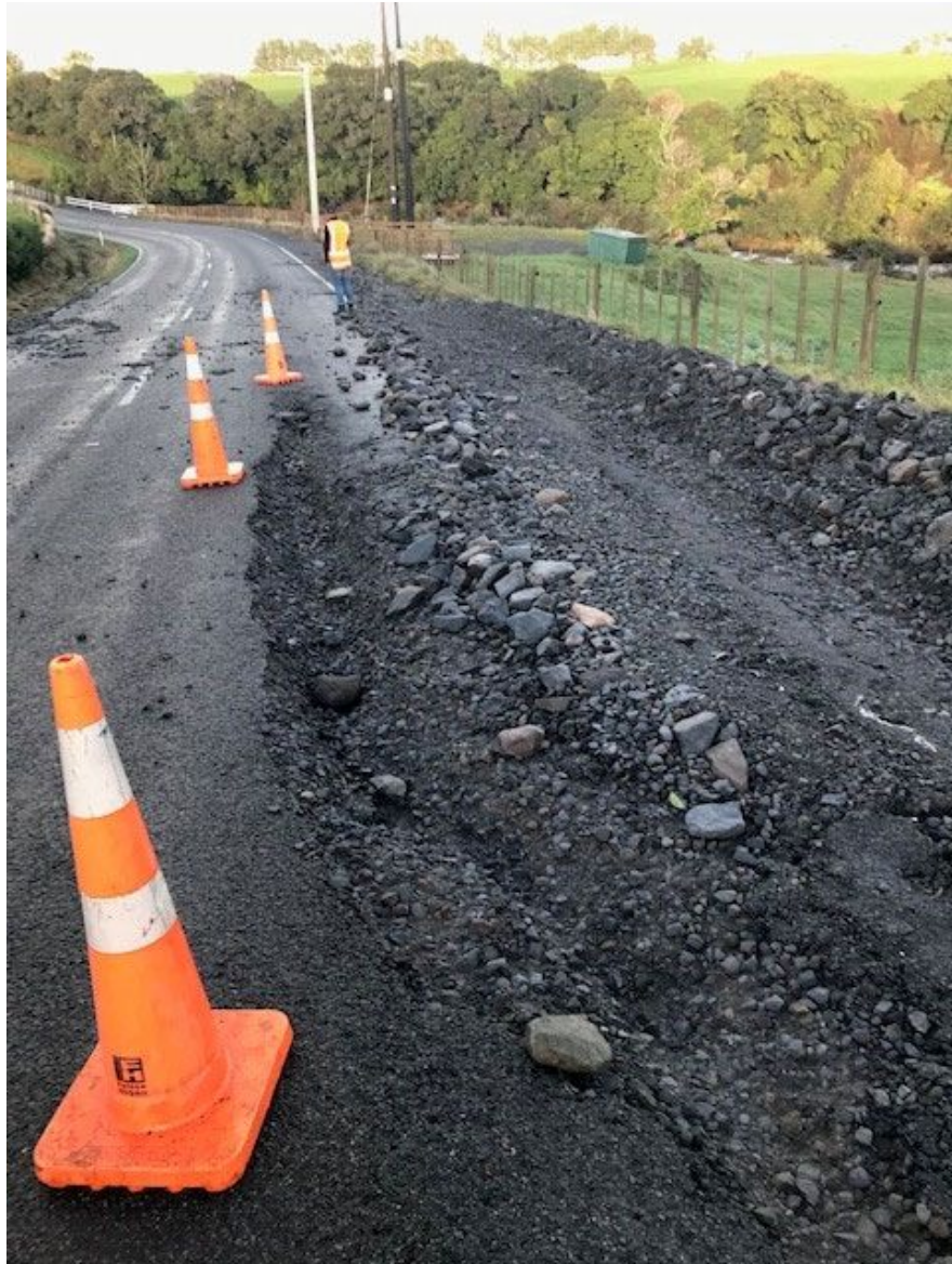
Figure 9: Palmer Road - By district boundary. Reconstructed the road, installed additional drainage and sealed the water tables. Total cost $206,000.
