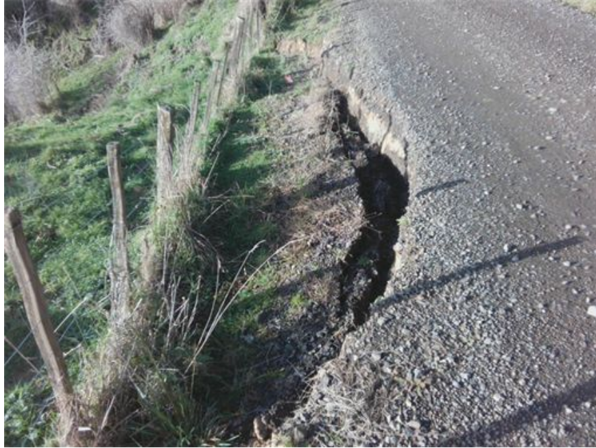
Figure 12: Whitianga Road RP1.35. As above, a retreat or a retaining wall. Estimated costs $30,000 - $75,000.
