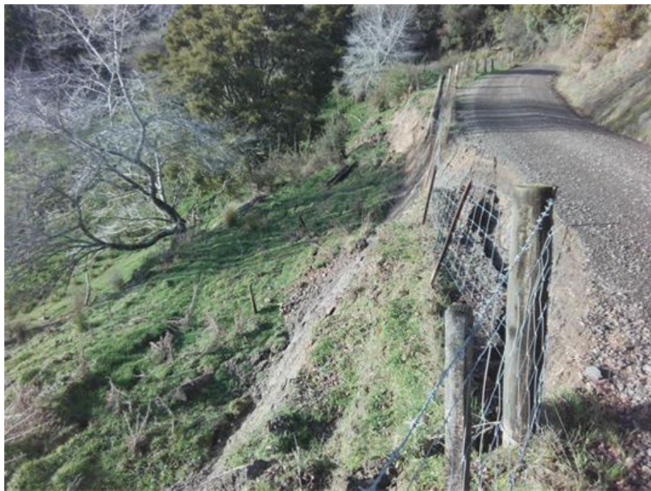
Figure 6: Whitianga Road RP0.92. As above a retreat or a wall. Please note the erosion further along the road immediately after the slip. Estimated costs - $30,000 - $100,000
