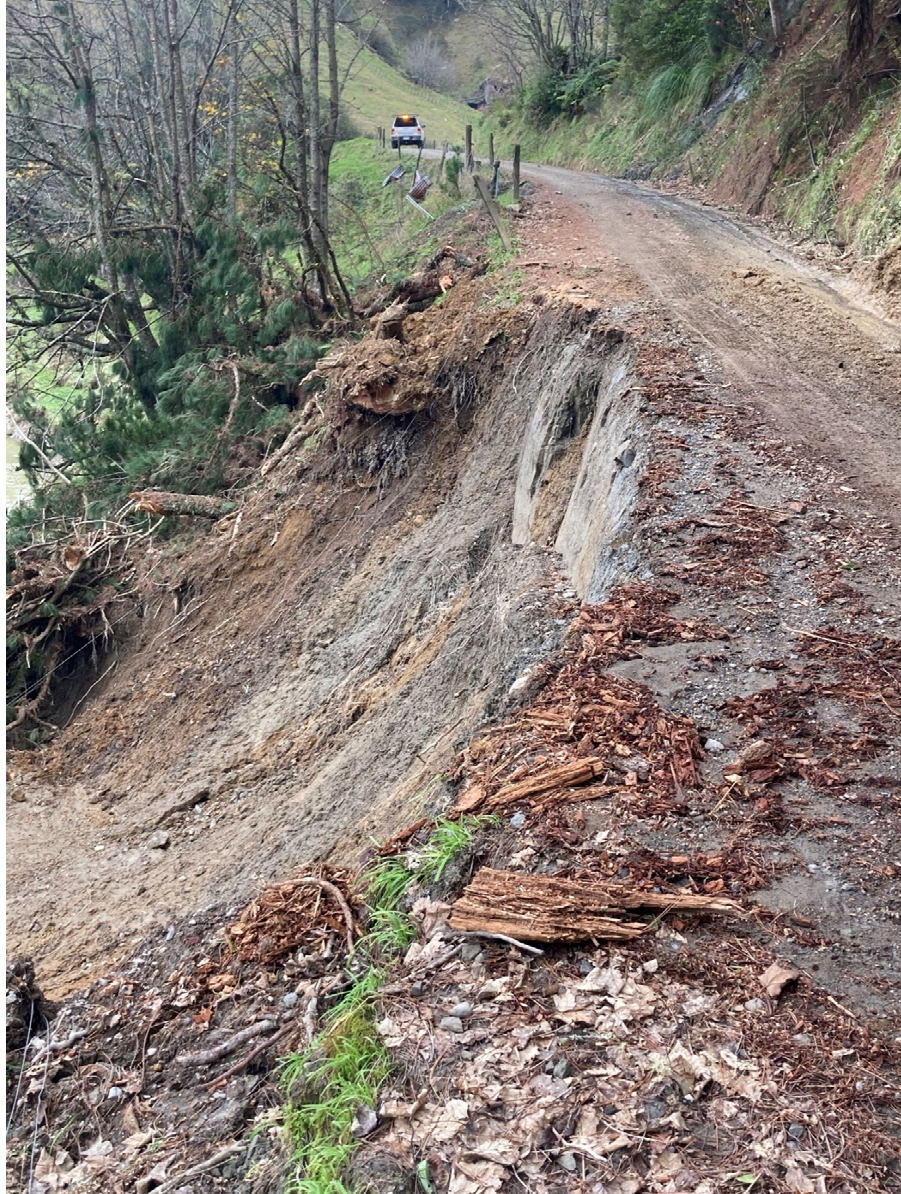
Figure 4: Whangamomona. Suggested treatment is a bank retreat to the right of the photo. There is a large macrocarpa tree which is leaning over the road which will need to be removed. This is being priced at present. Estimated to be in the order of $50,000 - $80,000.
