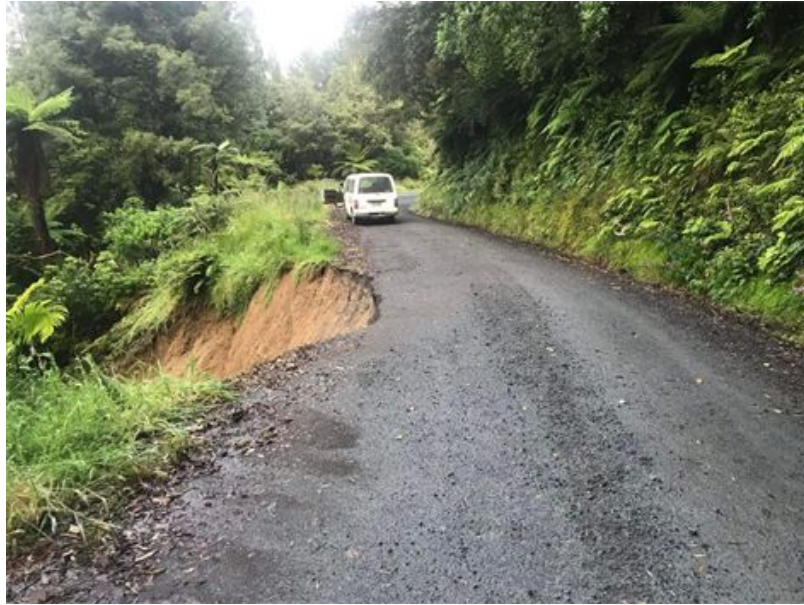
Figure 2: Junction Road. A similar treatment to Mangaoapa Rd, tied back retaining wall. Cost in the range of $50,000 - $75,000
