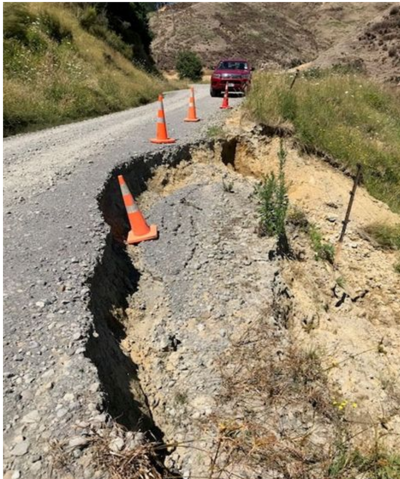
Figure 3: Douglas North Road. Suggested treatment a tied back retaining wall. Estimated cost $100,000 - $130,000
