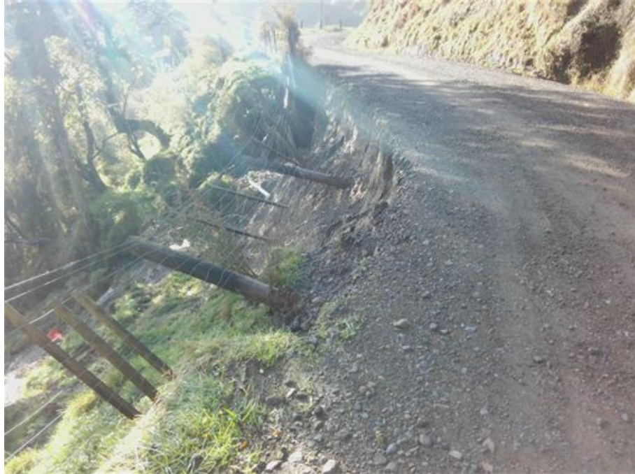
Figure 5: Whitianga Road RP0.58. Possibly a retreat or a retaining wall. To be confirmed. Estimated costs $30,000 - $75,000 depending on option chosen
