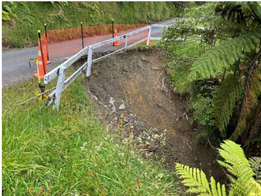
Figure 1: Mangaoapa Road. The suggested treatment is a tied back steel retaining wall. Estimated value $50,000 - $75,000
