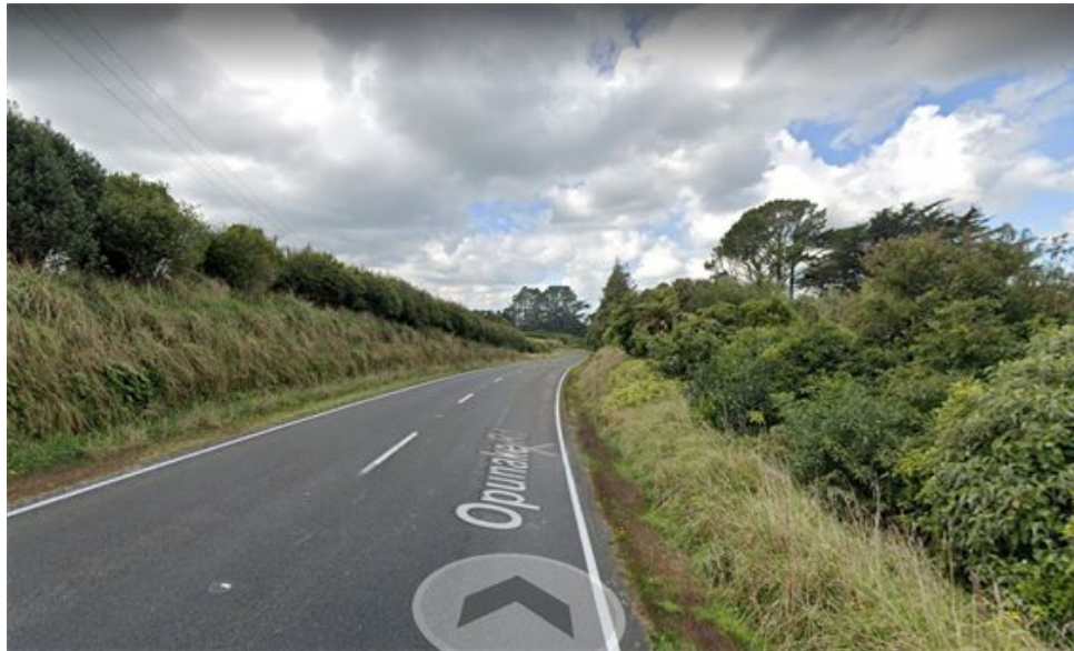
Towards Stratford from Mahoe at about 780 Opunake Road showing the bank which shadows the road in winter and can be icy going into the corner - no warning signs
