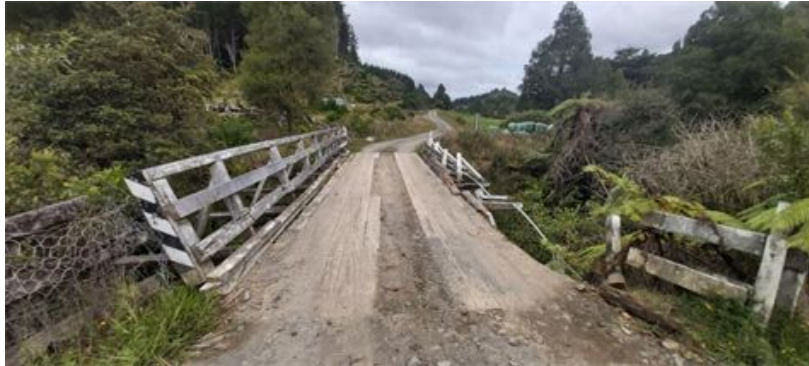
Figure 1: This damage was caused on 22 February 2022.
