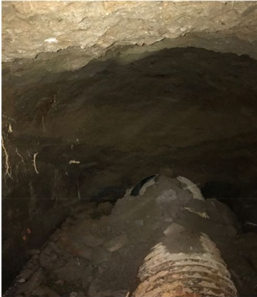
Figure 1 – Collapsed culvert under Manaia Road. This cavity is approximately 6m long x 1.5m high and 3m wide. Note the gap between the two culvert pipes at the joint.
