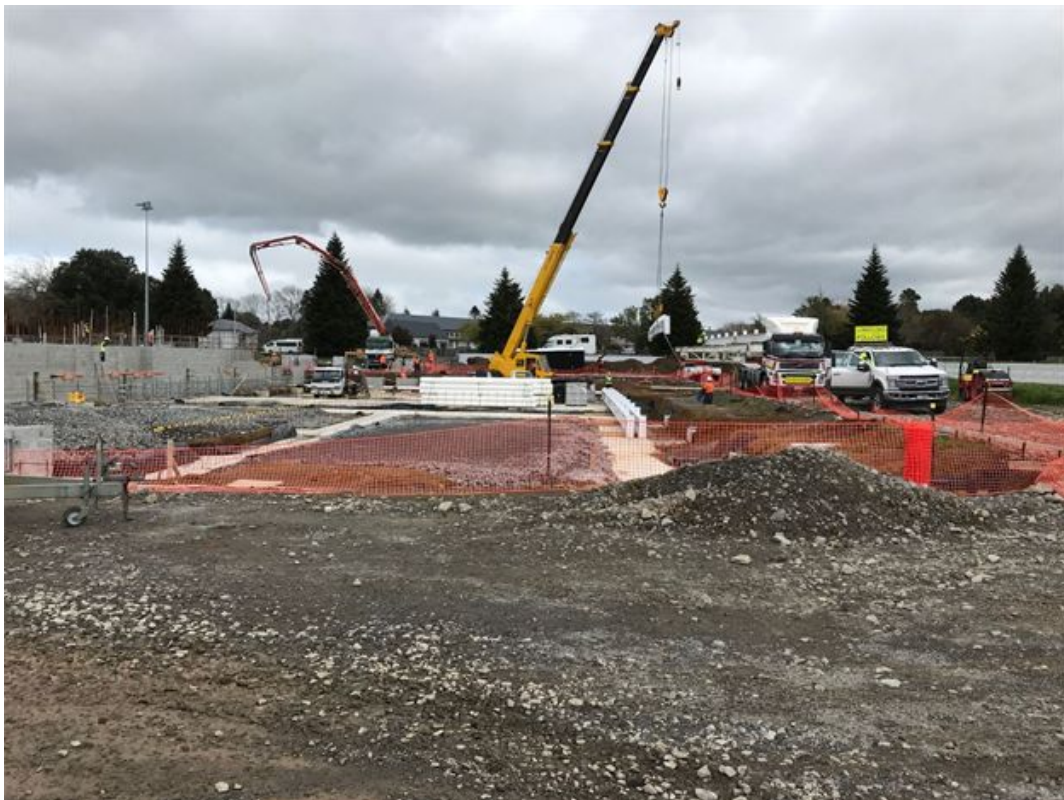
Figure 7: New aquatic centre dryside blockwork being filled and portal steel being lifted to site
