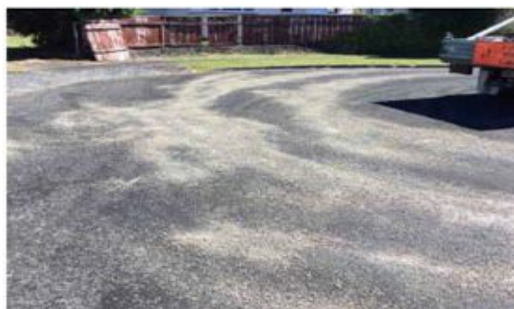
Figure 2 – Absorbent material spread on the bleeding bitumen.
