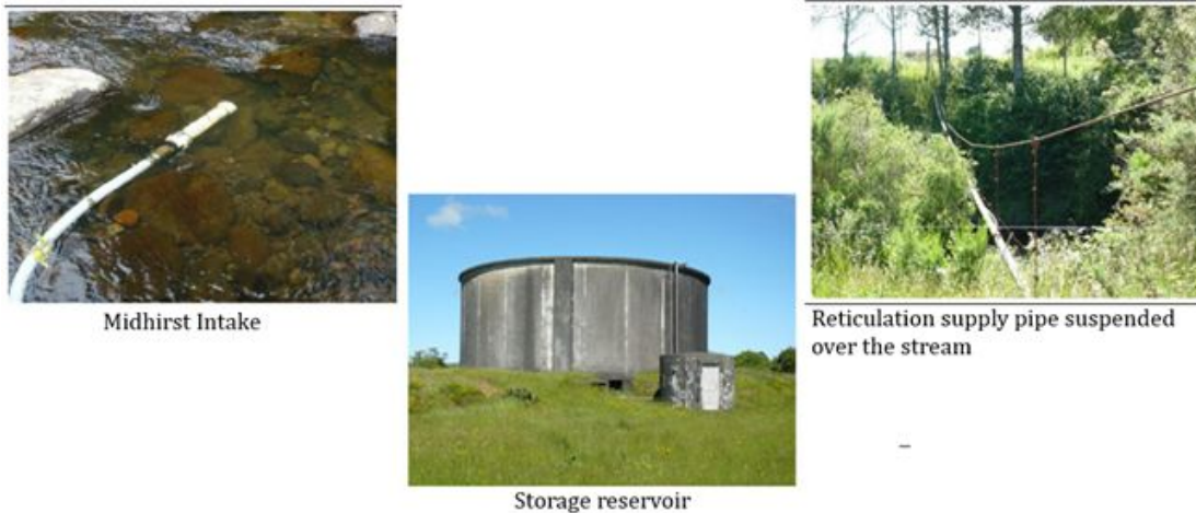
Figure 11 - Midhirst Water Plant Photos
