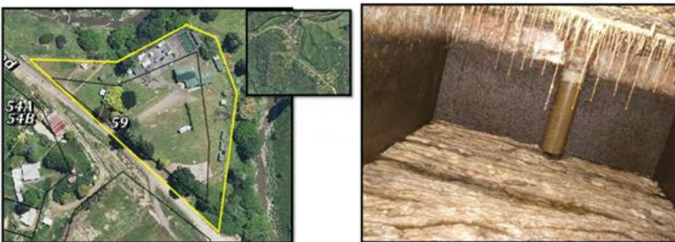
Figure 30 - Whangamomona Septic Tank and Fat Build Up
