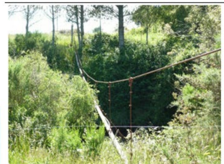
Reticulation supply pipe suspended over the stream
