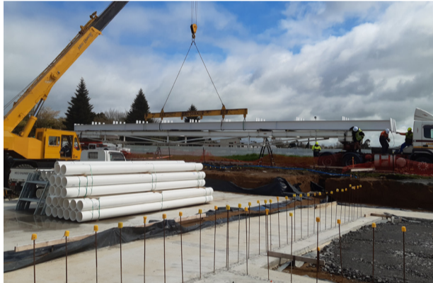
Framing for the Aquatic Centre Development is craned onto the construction site on 1 October 2021.
