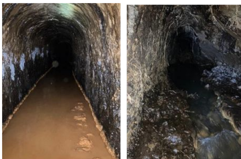
Figure 8: Stormwater Tunnels - Juliet Street & Pembroke Road
