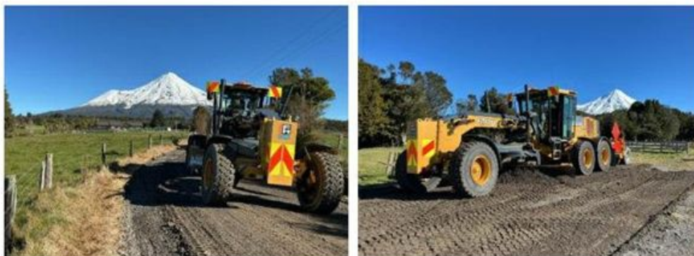
Figure 1: Footpath, edge breaks and grading
