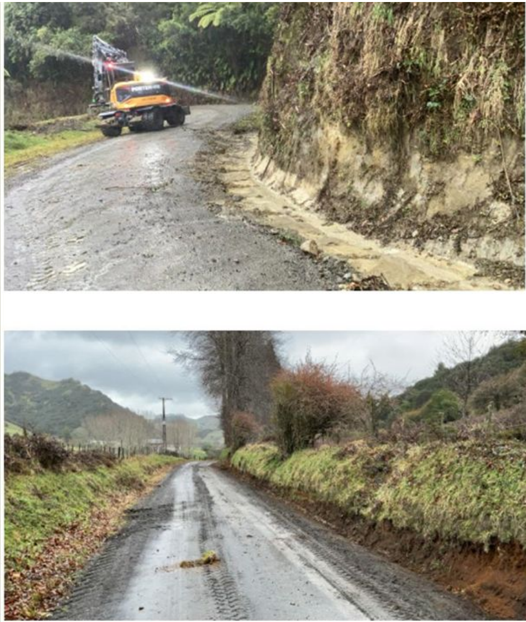
Figure 3: Upper Mangaehu Road water tables
