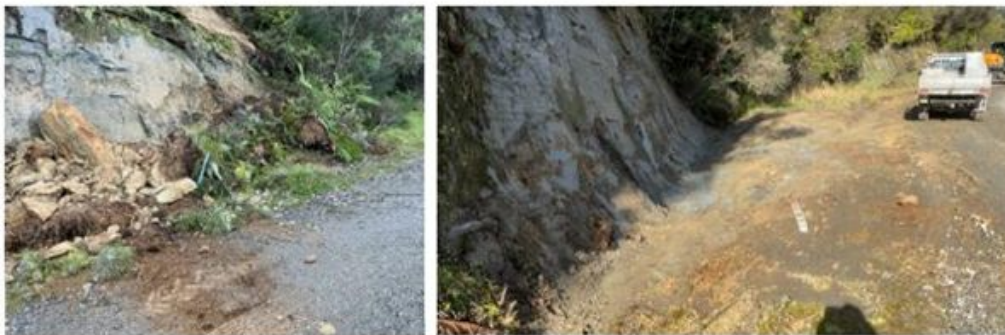
Figure 2: Surfacing, drop outs, slips
