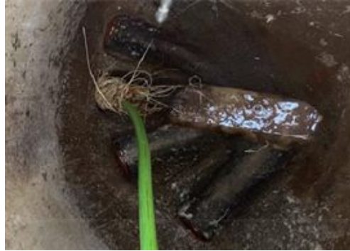
Figure 6: Macerated Roots Blocking Sewer Lateral
