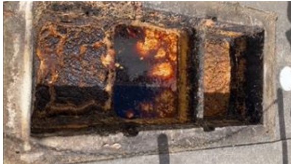
Figure 7: Odorous Grease Trap – Portia Street
