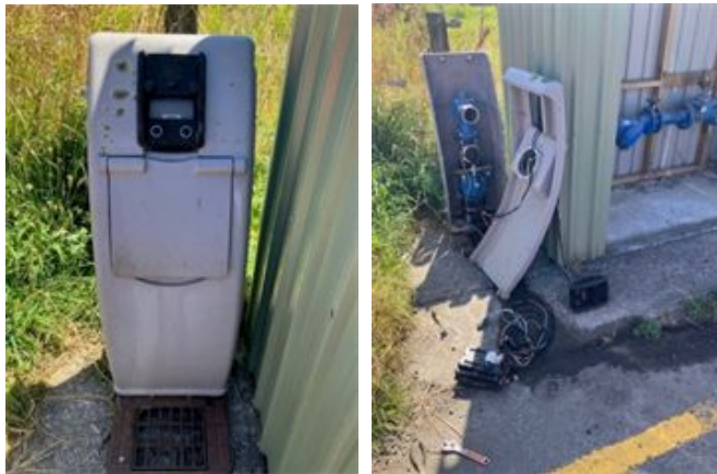
Figure 5: Inoperable hydrant unit and subsequent repair
