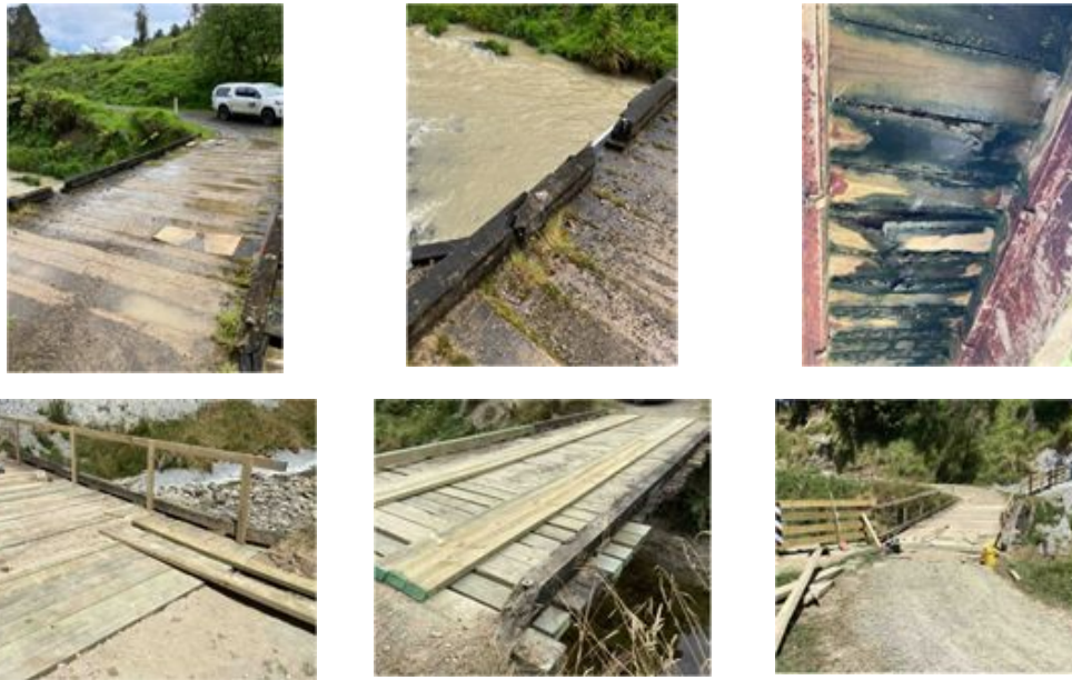
Figure 1: Gowers Access Bridge - Damage and Repairs.
