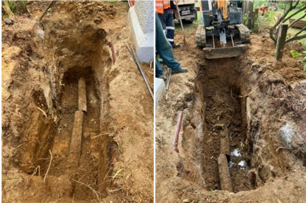
Figure 6: Unearthed broken sewer pipe
