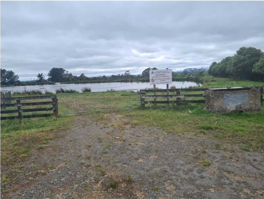
Figure 5: The current access gate to the wastewater oxidation pond, there is no electrified wire on the fence.
