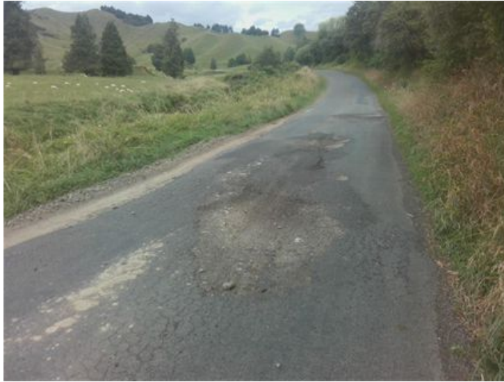
Figure 2: Damage to Brewer Road
