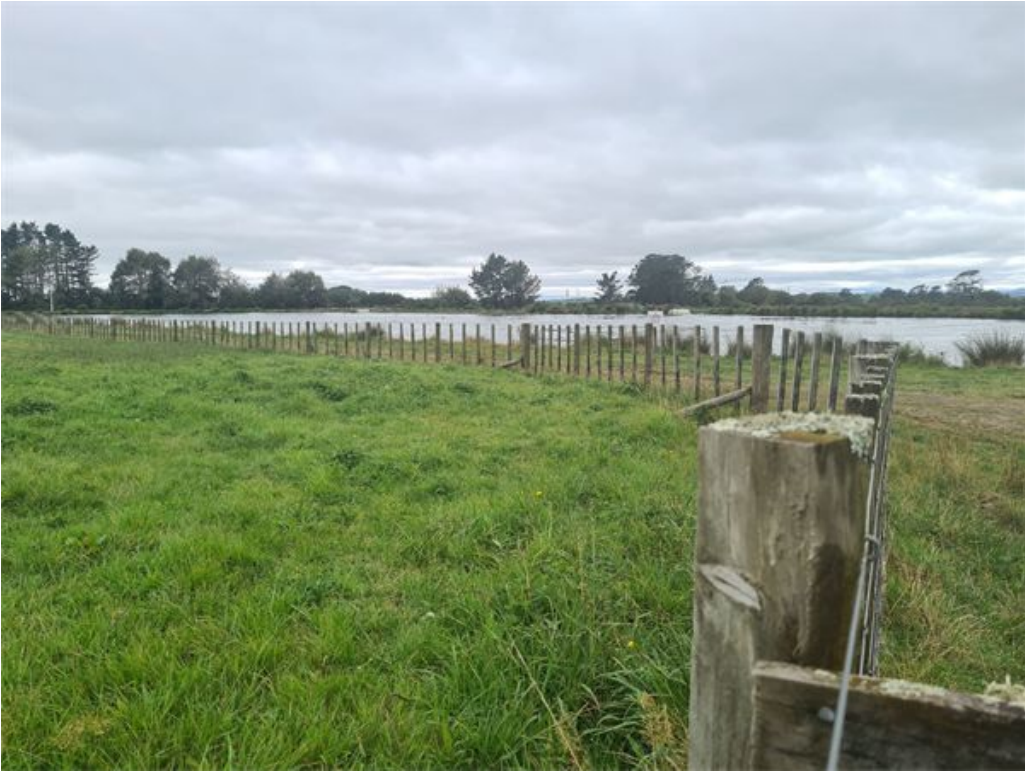
Figure 6: A portion of the current stock fencing around the oxidation pond, there is no electrified wire on the fence.
