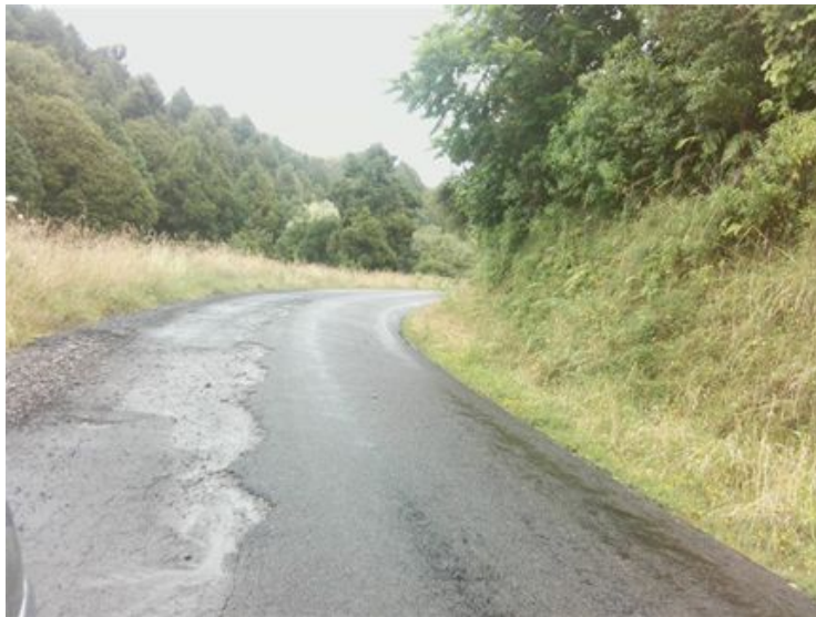
Figure 1: Just one of many patches to be repaired on Mangaehu Road.
