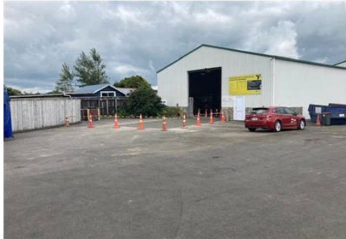
Figure 6: Completion Photo of the concrete apron out the front of the Transfer Station Shed
