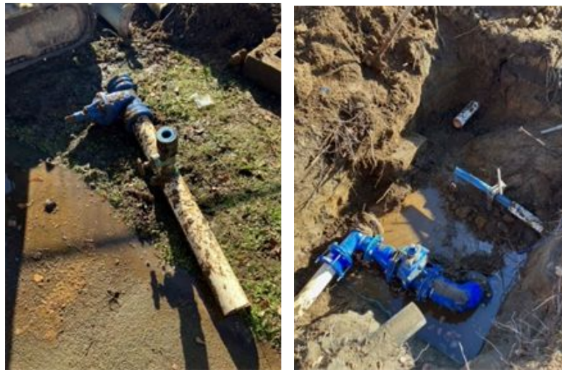
Figure 5: Broken push-fit valve
