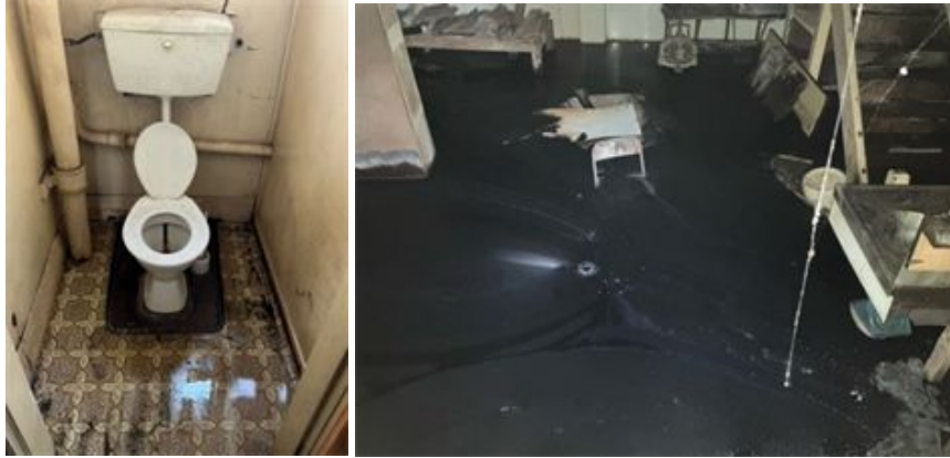
Figure 6: Leaking toilet cistern and flooded basement (submerged chair in centre)
