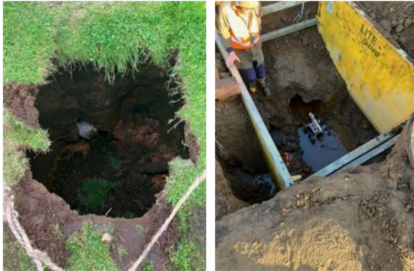
Figure 8: 10' deep sinkhole and excavation prior to camera assessment
