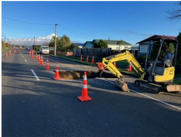
Figure 7: Pembroke Road - lane closure due to collapsed sewer pipe
