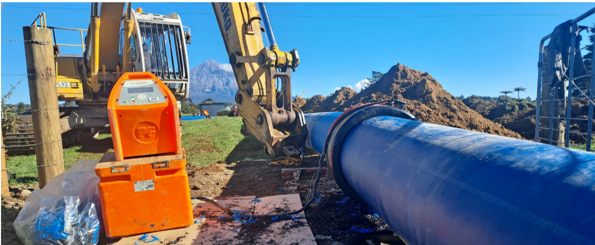
Significant progress on the second water trunk main between the Stratford water treatment plant and Stratford township.
