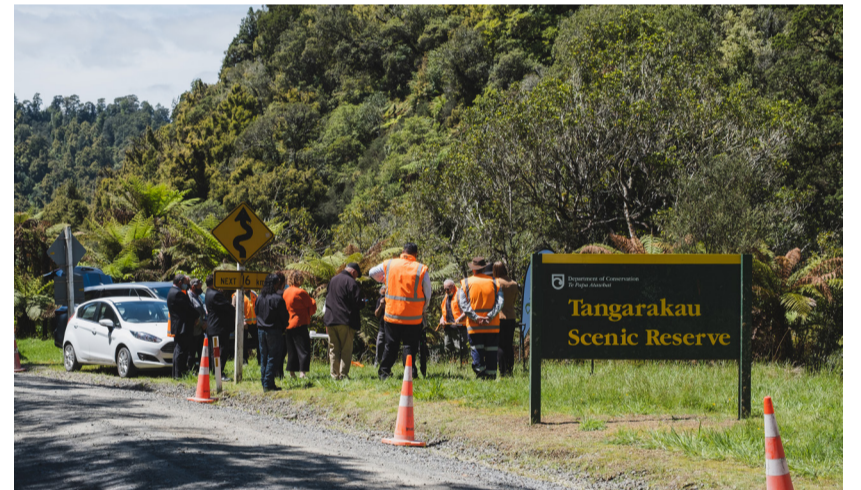
Sealing work progressing on the historically unsealed stretch of State Highway 43 along with a suite of other safety improvements.
