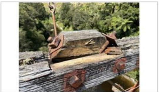
Cracked cross brace block in handrail truss
