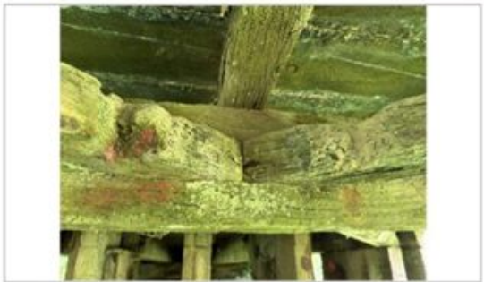
Deteriorating cross members
