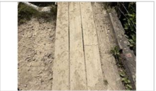
Cracked running board
