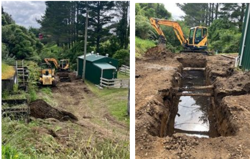
Figure 9: Midhirst WTP Backwash Soakage Field
