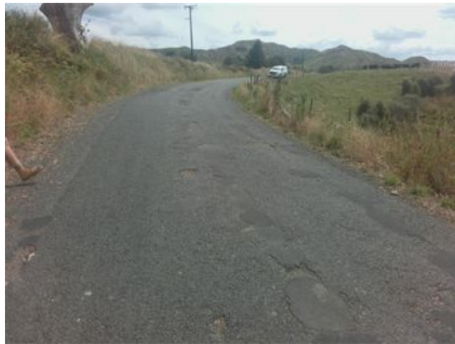
Figure 3: Damage to Mangaotuku Road
