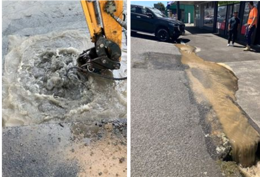
Figure 10: Miranda Street and Broadway Rider Main Leaks
