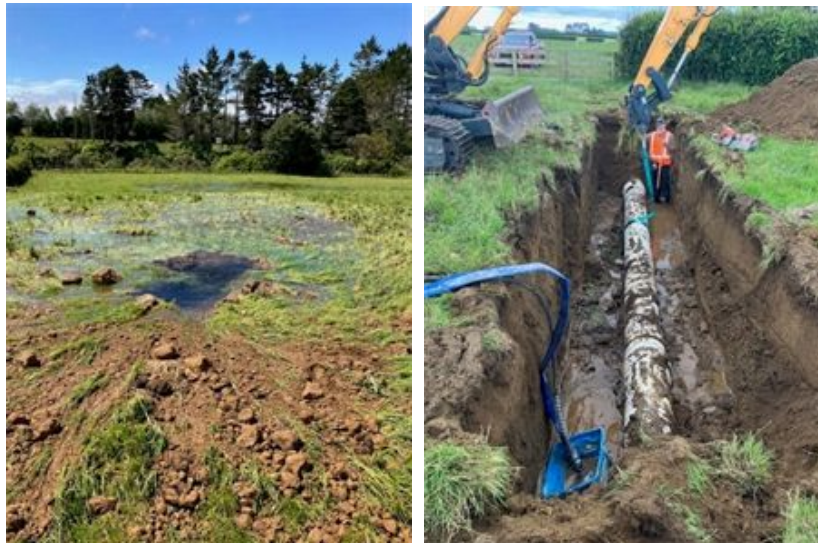
Figure 11: PVC Trunk Main Break
