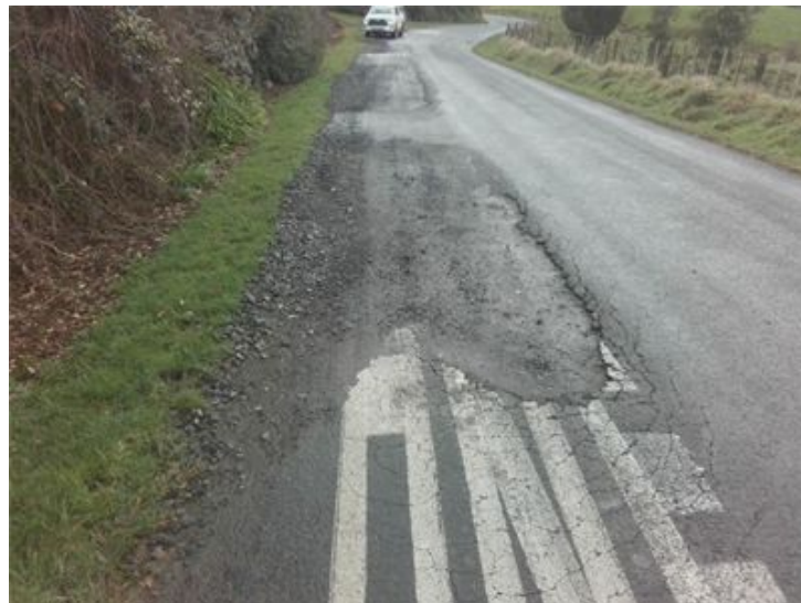
Figure 4: Damage to Brewer Road
