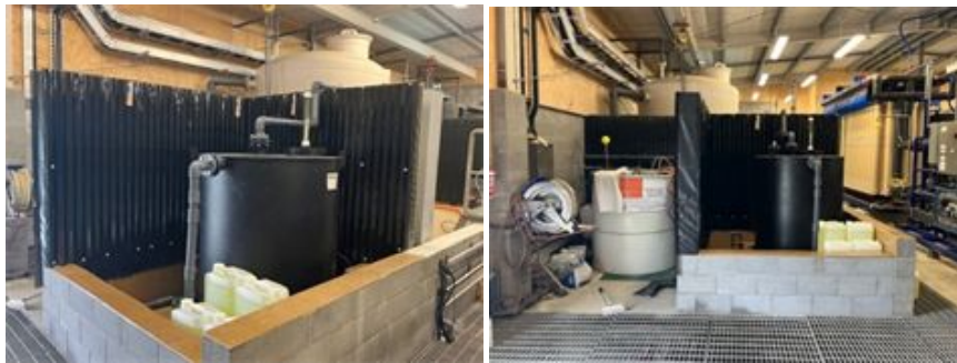
Figure 8: Sodium Hypochlorite Bund
