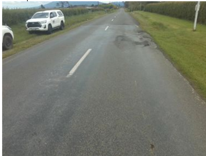
Figure 1: Damage to Beaconsfield Road
