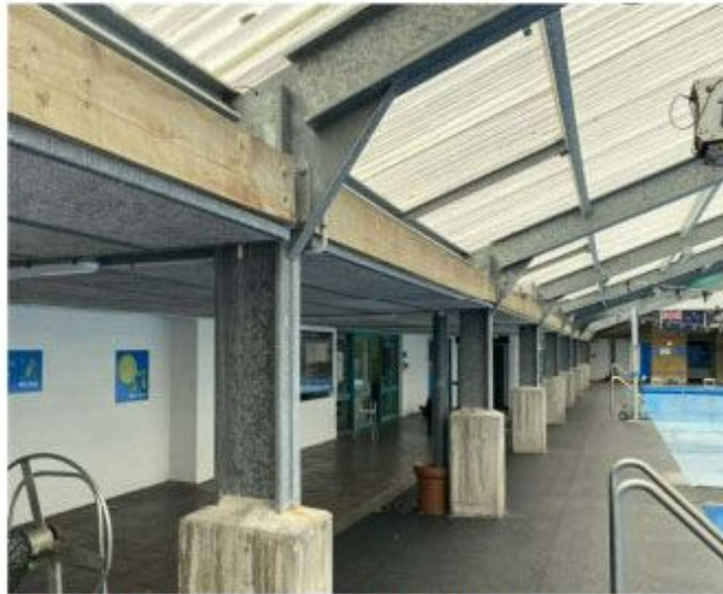
Figure 3: North side of portal frame structure (note lack of braces). Possible portal frame action between bays.
