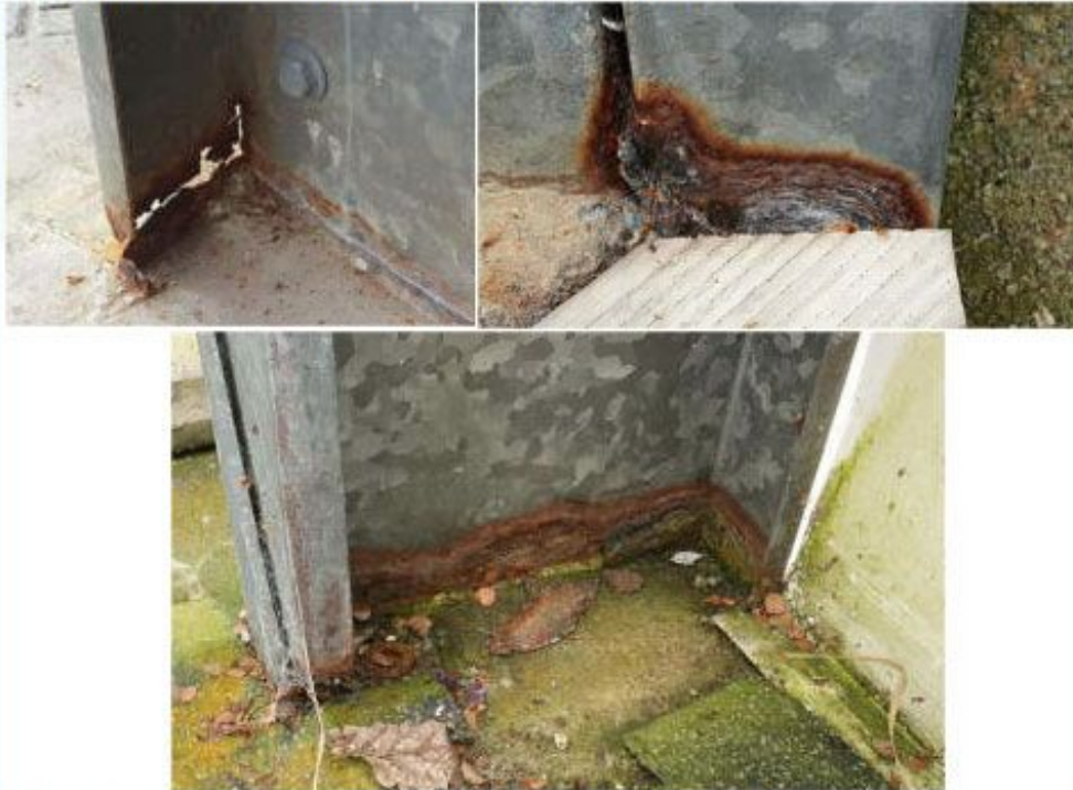
Figure 5: Photos showing severe corrosion at the base of the portal frame columns.
