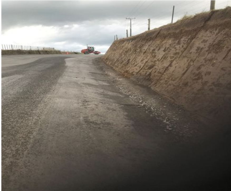
Figure 3: Palmer Road being prepared for sealing. Note the shape of the water table as this is to be sealed also to prevent further scouring.
