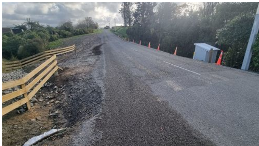
Figure 1: Monmouth Road open to traffic. A sight rail is to be installed where the cones are located.
