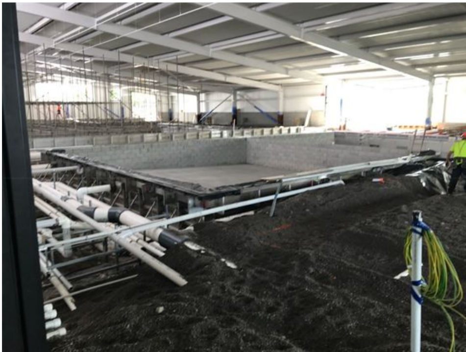
Figure 13: Aquatic Centre internal showing learn to swim and programmes pools in centre and toddler pool and splash pad foundation work in foreground.
