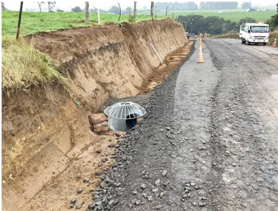
Figure 2: Drainage catchpit and bank trim on the eastern side of Palmer Road.
