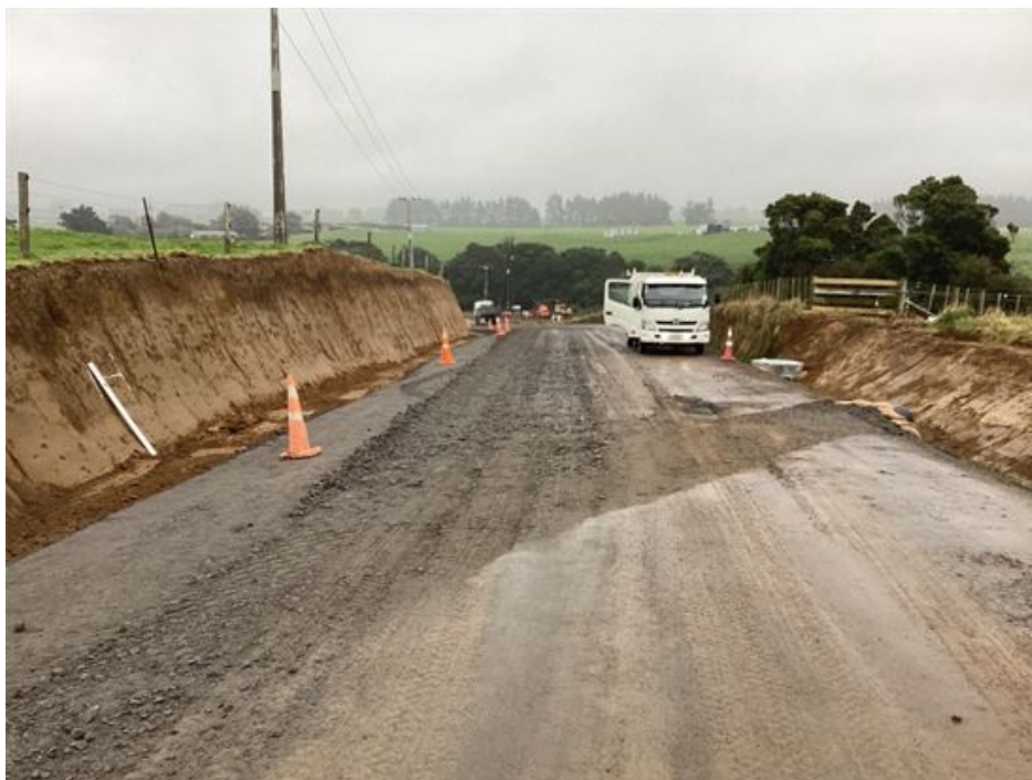
Figure 5: Palmer Road being reconstructed. Note the culvert trench across the road and the new catchpit on the southern side of the road
