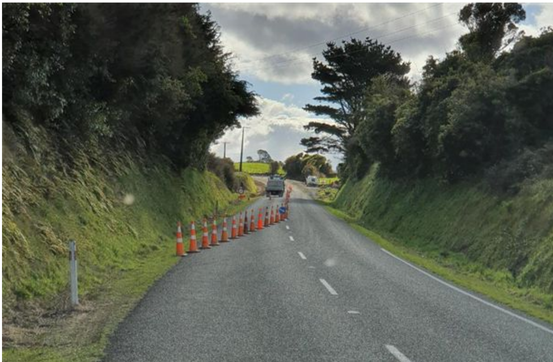
Figure 14: Example of good TTM – Opunake Road lane closure to enable safety improvement works
