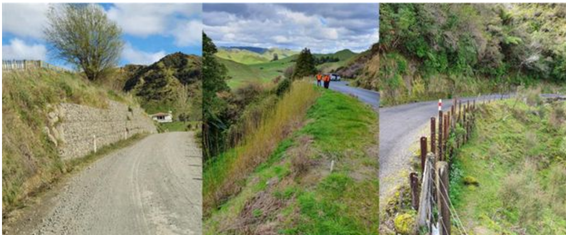
Examples of retaining wall applications. Left: gabion wall (Mangaehu Road). Centre: living wall (Brewer Road). Right: old post (railway iron) and panel wall (Mohakau Road).
