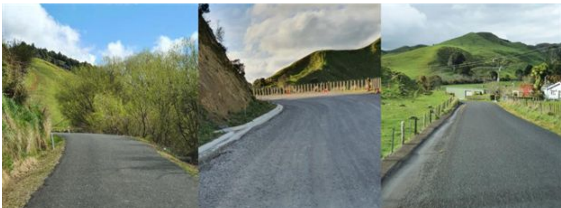
Examples of effective drainage. Left: Unlined water table drain (Mokahau Road). Centre: new K & C constructed in conjunction with pavement rehab works (Mangaotuku Road). Right: concrete channel to prevent table drain scour during high rainfall events (Makuri Road).
