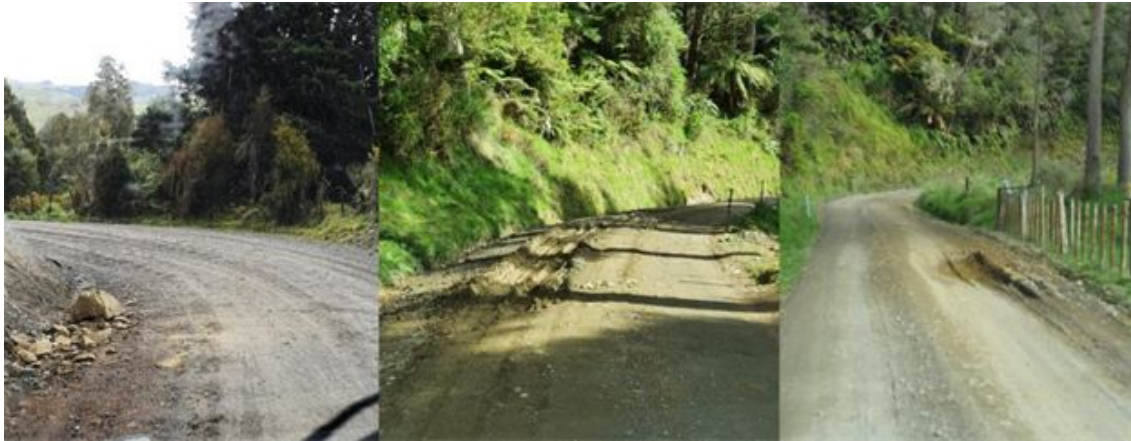
Examples of logging truck damage. Left: Corrugated road surface caused by higher vehicle stresses (Junction Road). Centre & Right: Deep pavement failures resulting from insufficient pavement strength for additional logging truck loading (Puniwhakau Road).
