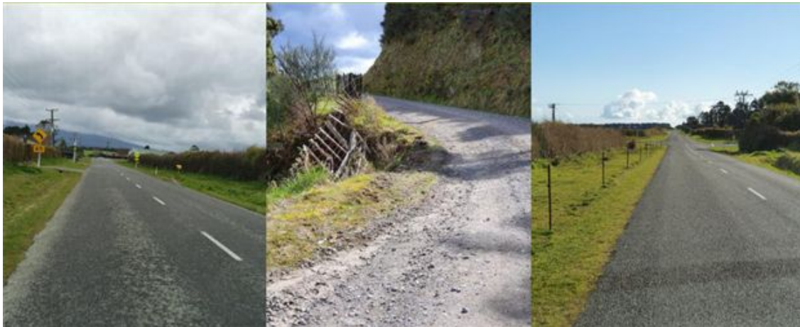
Examples of rural road safety issues. Left: Pembroke Road - incorrect curve advisory sign and poor delineation. Centre: Junction Road - drop-out without delineation or bund to limit water infiltration. Right: Opunake Road - temporary fence with waratah standards installed on road berm
