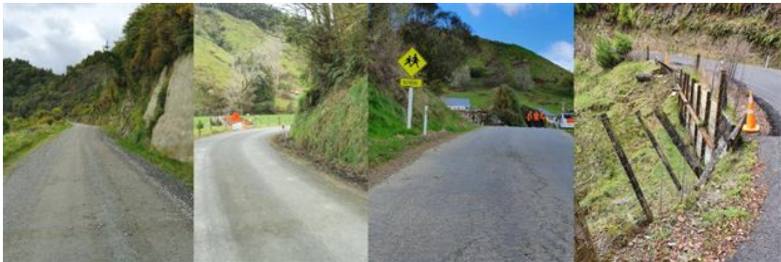
Examples of ineffective rural drainage. Left: substandard water table drain maintenance on Junction Road and Makuri Road (common throughout rural network). Right: ineffective water table drainage contributing to premature road pavement failure (Brewer Road) and ineffective asphalt bund allowing water infiltration and the need to extend retaining wall (Mokahau Road).
