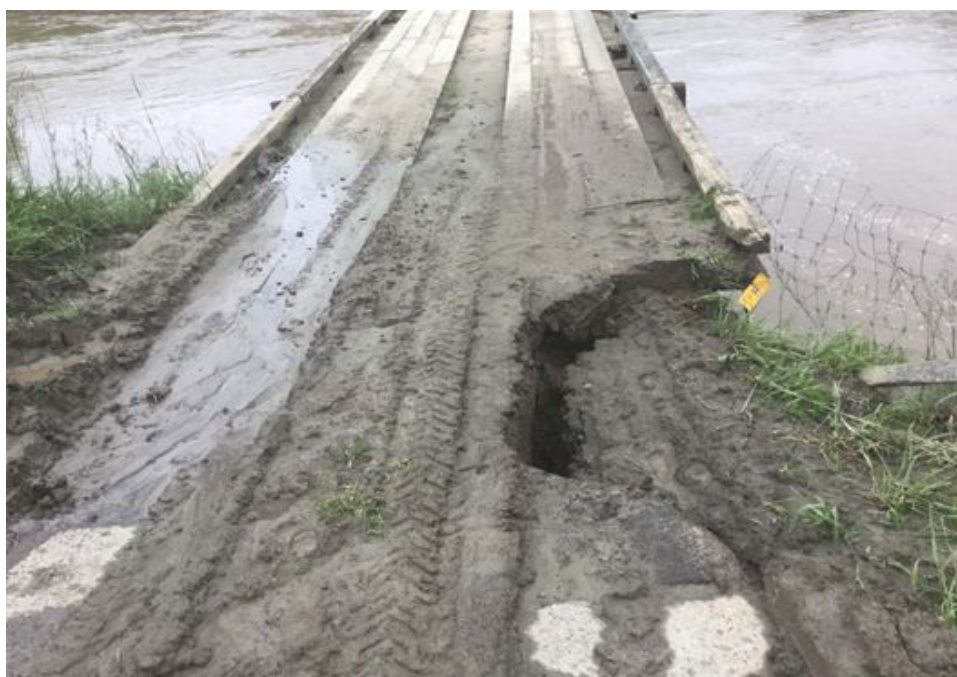
Figure 1: Further Damage to McBride's Bridge
