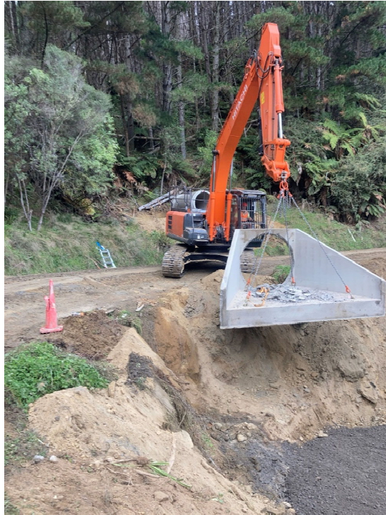
Figure 3: Lowering the headwall into place at the outlet of the new culvert.
