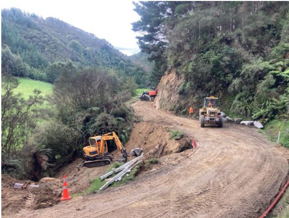
Figure 2: Preparation of foundation for the outlet headwall. Note, the existing water drive is indicated by the culvert marker post
