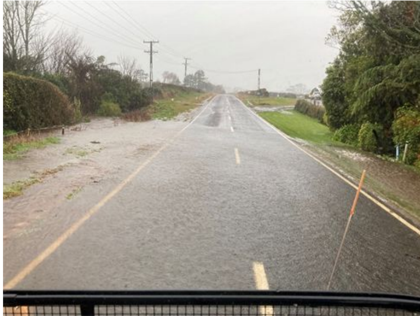
Figure 4: Flood water running across Opunake Road
