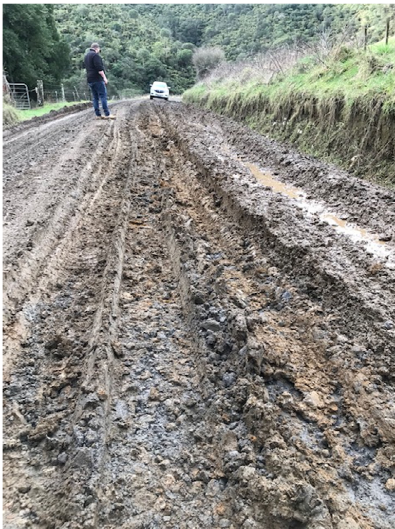
Figure 5: One of the large areas of road damaged. This hole is 50m long x 2.5m wide
