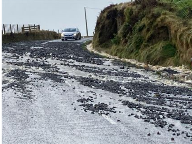
Figure 2: Gabion rock strewn across Palmer Rd that was washed out of roadside drain
