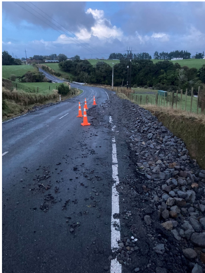
Figure 3: Rock blocking drain which lead to the road being scoured out
