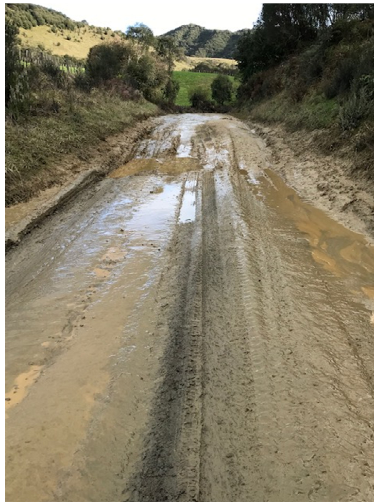
Figure 6: This hole is the full width of the road and 600mm deep
