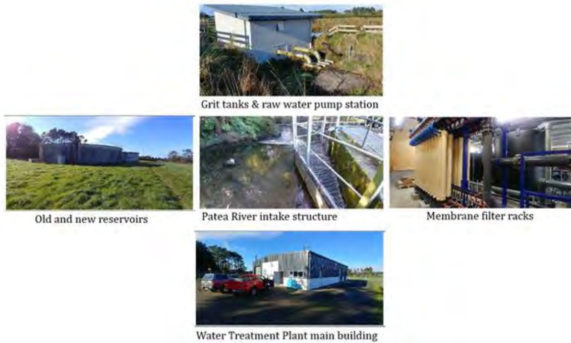
Figure 9 - Stratford Water Treatment Plant Photos
