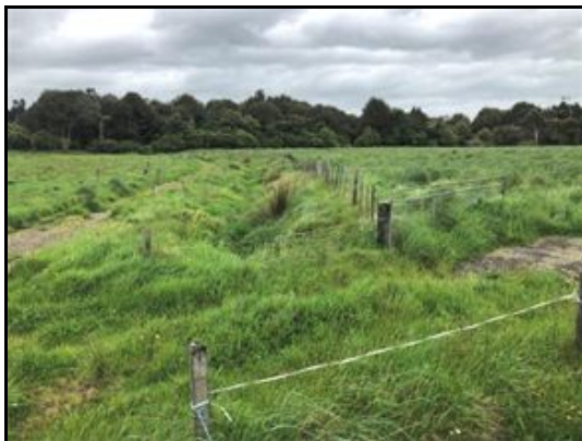
Eastern open drainage system
