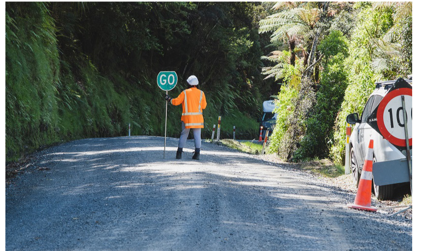
Sealing of State Highway 43 was confirmed and has since started in late 2021.
